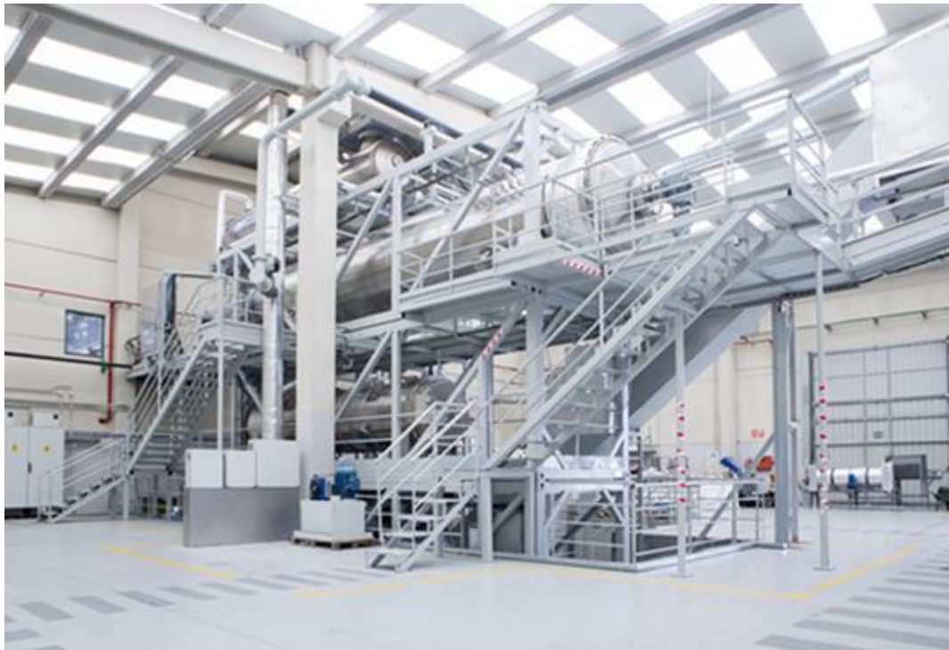
BIOMAK - Industrial Thermal Hydrolysis unit. ECONWARD's facilities (Rivas Vaciamadrid, Spain)
