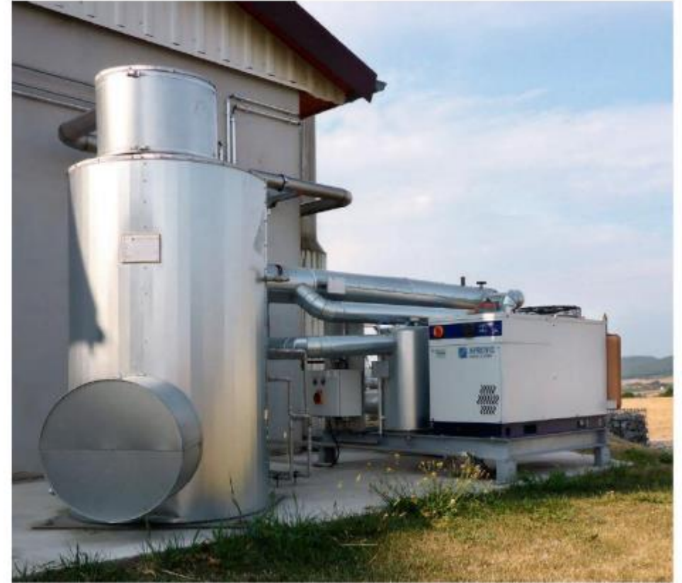
External insulated desulphurisation-unit (activated carbon) and cooling unit for dewatering
