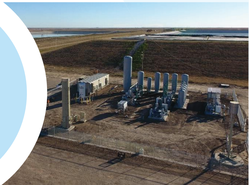
Warrior Wastewater Treatment Plant Biogas Project — City of Dodge City, Kansas
